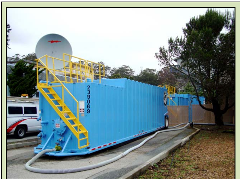
Baker Tanks located at Portola Pump Station, freshly painted and ready to go!
