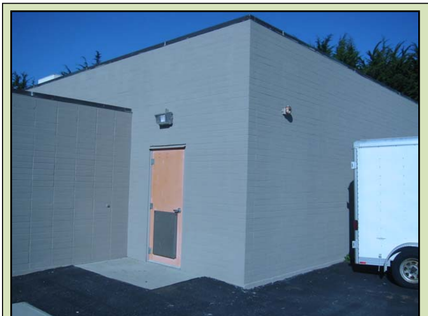
The Southern walls were sealed with a new coating color coded to the underlying masonry.
